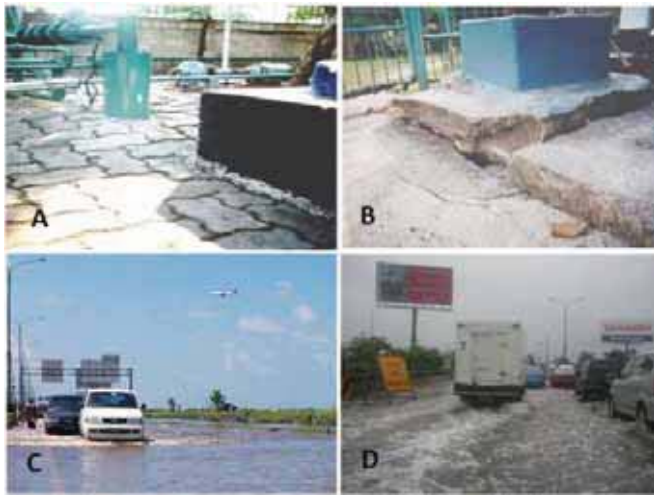
Figure 11. Several indication and impact of land subsidence in Jakarta [Wirakusumah, 2008]. A and B are locations in Kamal Muara; C and D are locations along the highway to the airport (Cengkareng).
