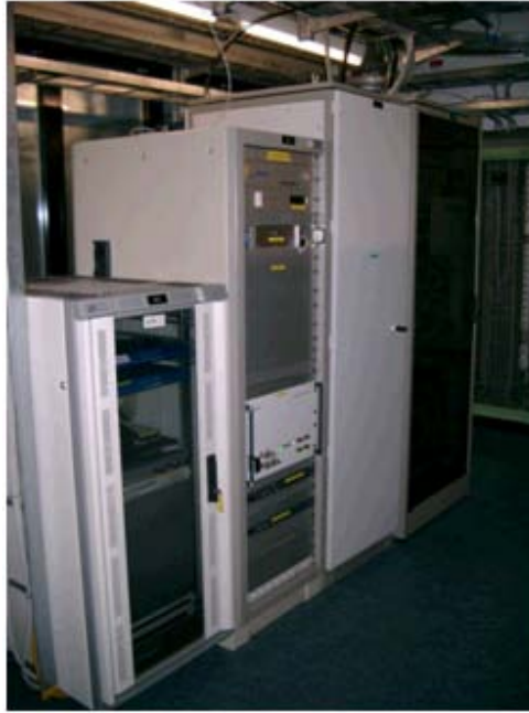
Figure 4.40: RIMS and WAN racks at Zurich airport
